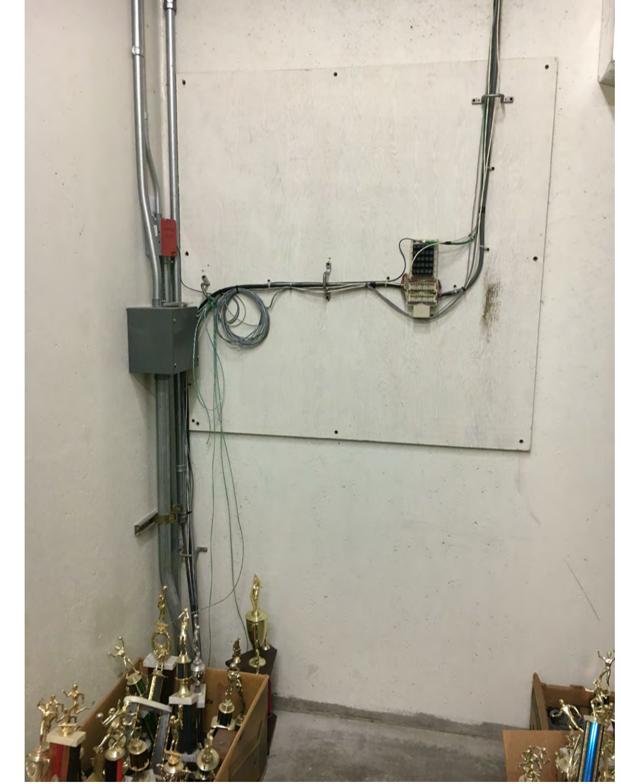
4 EXISTING LOW VOLTAGE TERMINATION BOARD ED1.3B SCALE: NTS
