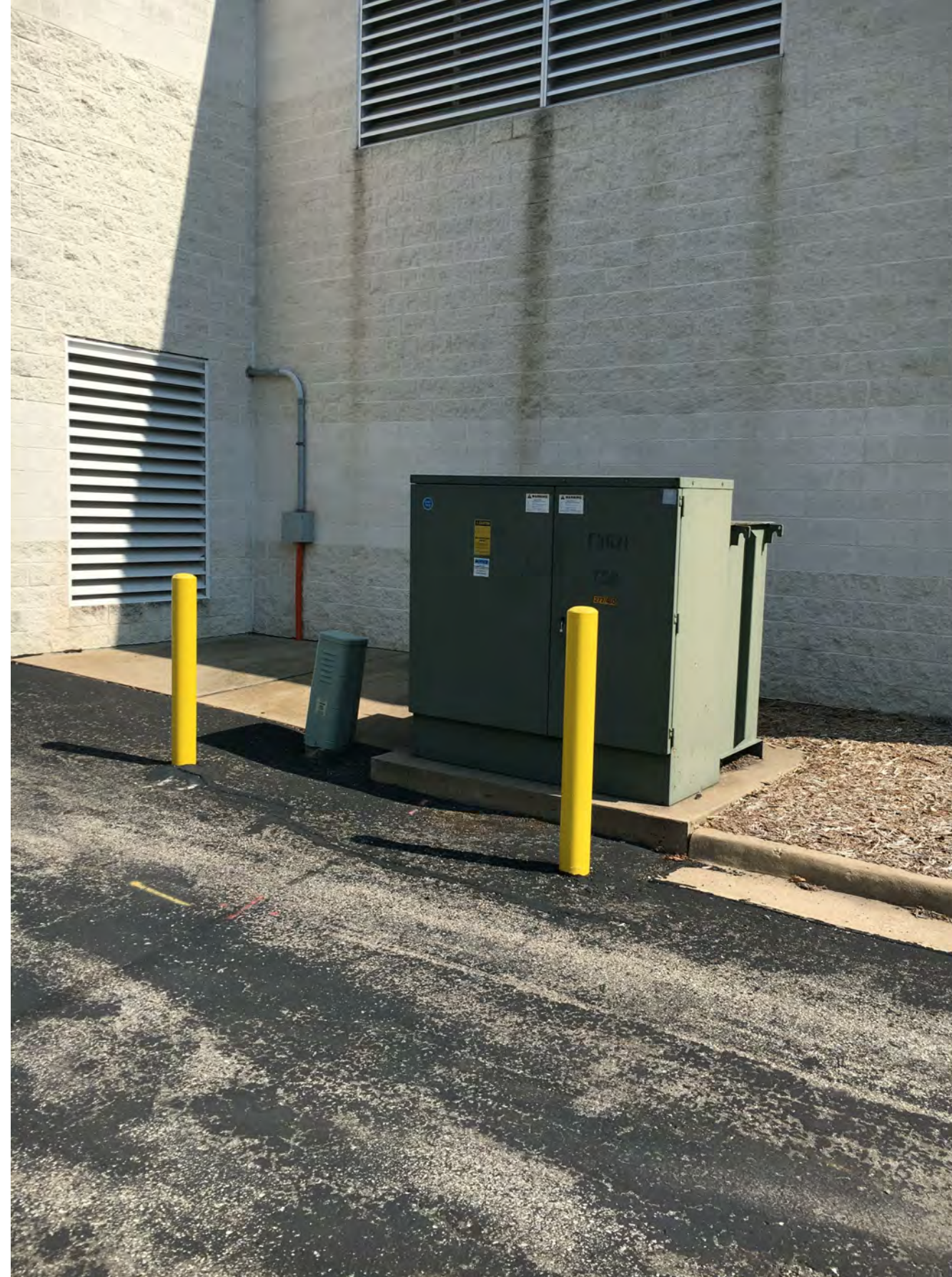
1 EXISTING SERVICE TRANSFORMER FOR SWITCHBOARD MDP-A SCALE: NTS
