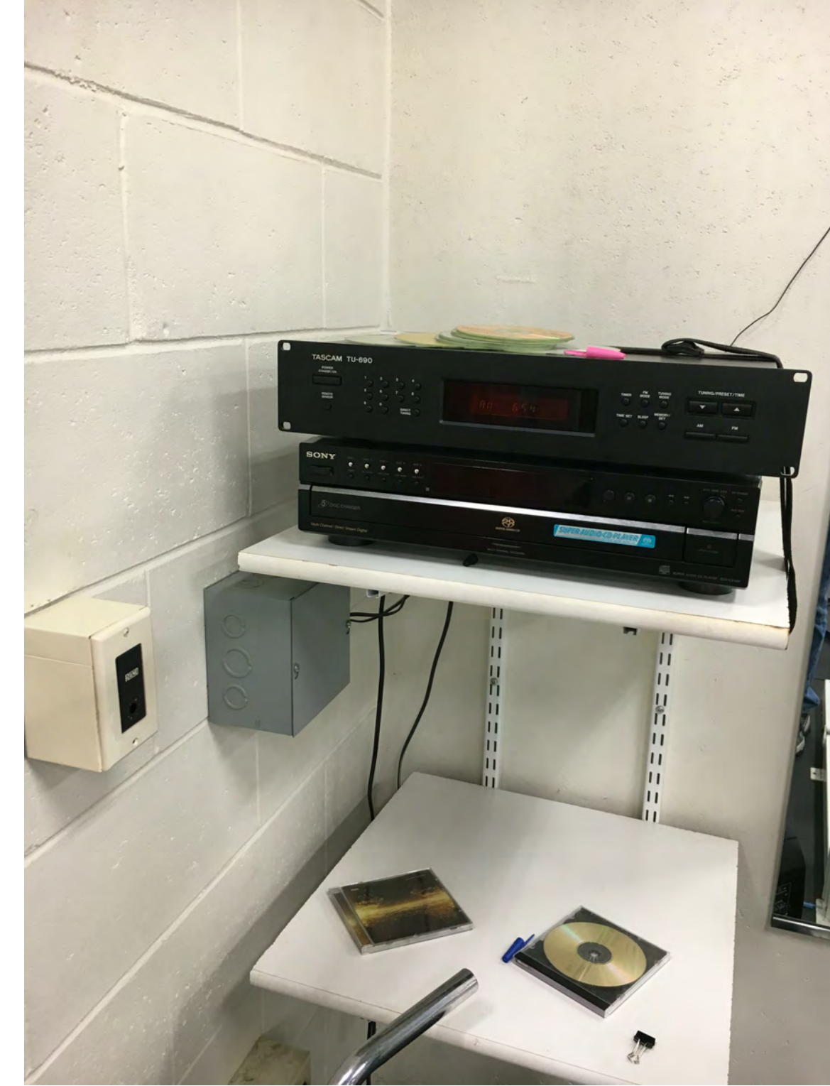
3 EXISTING WIEGHT ROOM CD AND TUNER FOR SOUND SYSTEM ED1.3B SCALE: NTS
